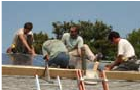
Expert installers and trainees fasten PV panels to a local rooftop. (Source: Anju Rajani)
