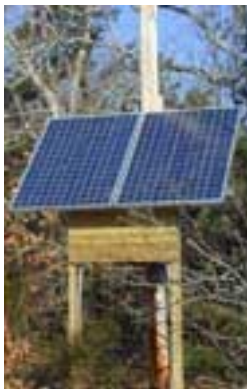
PV panels power a new system that lights up the trails at WBNERR's visitor center
