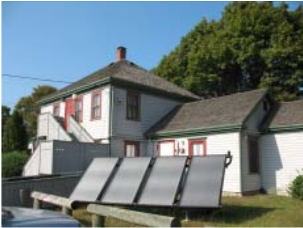
Solar thermal panels at Waquoit Bay Reserve
